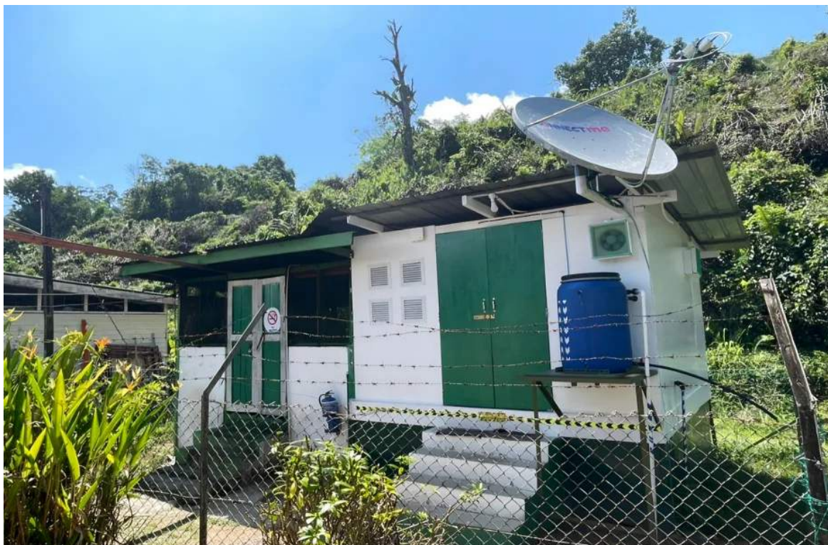
Figure 6-2 H2E System Powerhouse at Long Loyang Clinic
