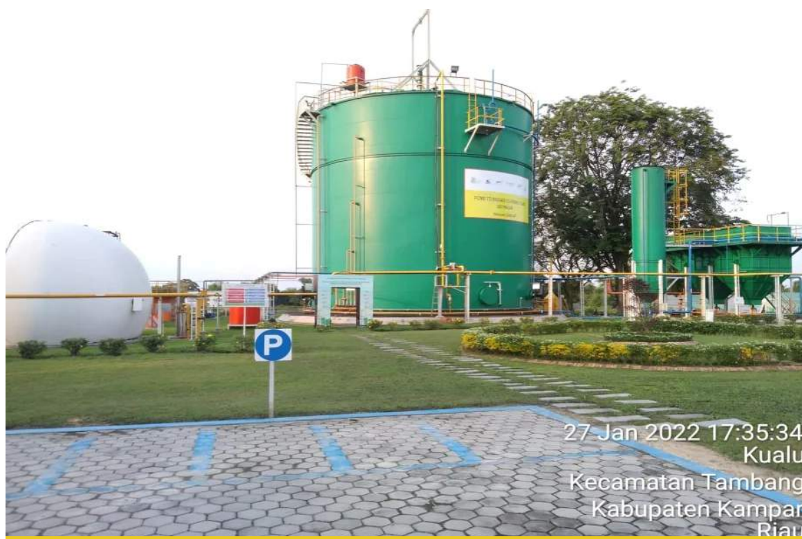
Figure 5-3 Biogas Cofiring Boiler at Sei Pagar POM
