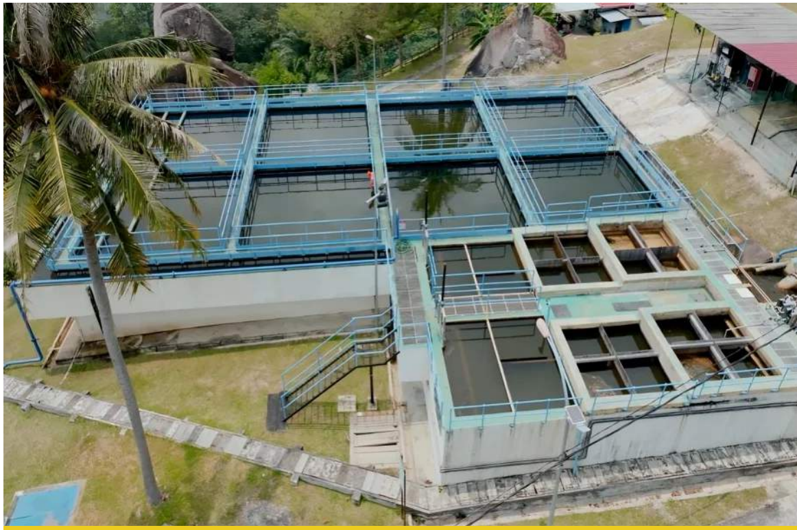
Figure 3-2 The Gunung Ledang Water Treatment Plant
