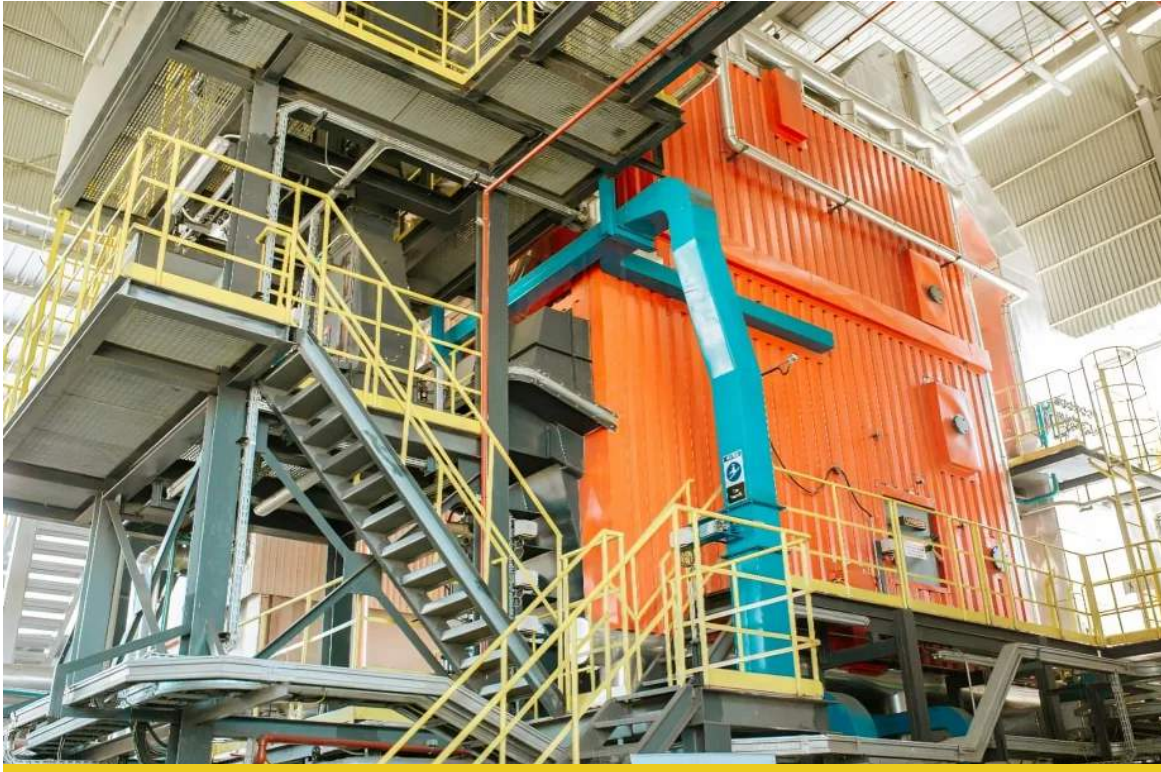
Figure 3-6 Biomass Boiler at Prambanan Factory Site
